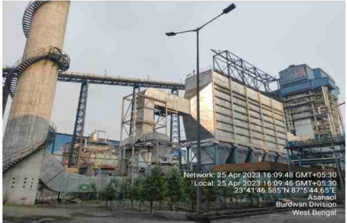
5 Field ESP for CFBC Boiler
