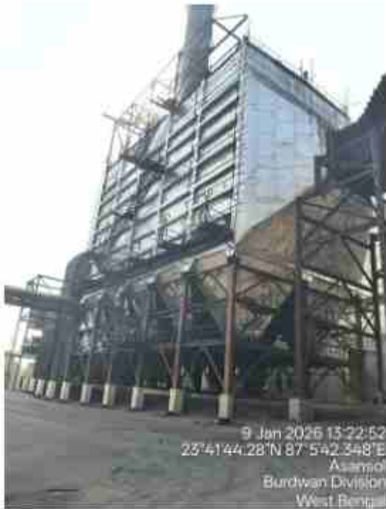
5 Field ESP connected with DRI through WHRB
