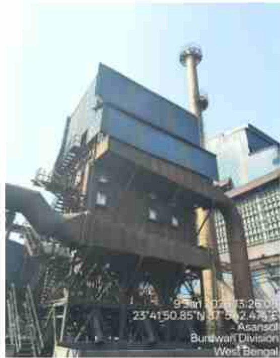
Bag Filter attached with Cooling Tower for DRI
