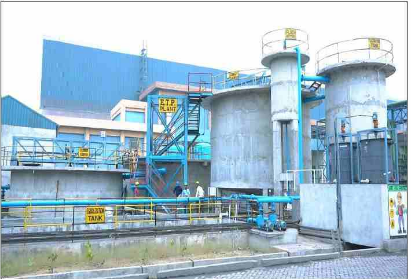
Effluent Treatment Plant (1540 KLD)
