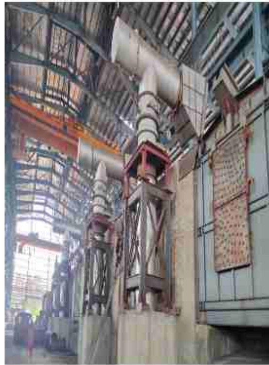
Induction furnace connected with primary hood
