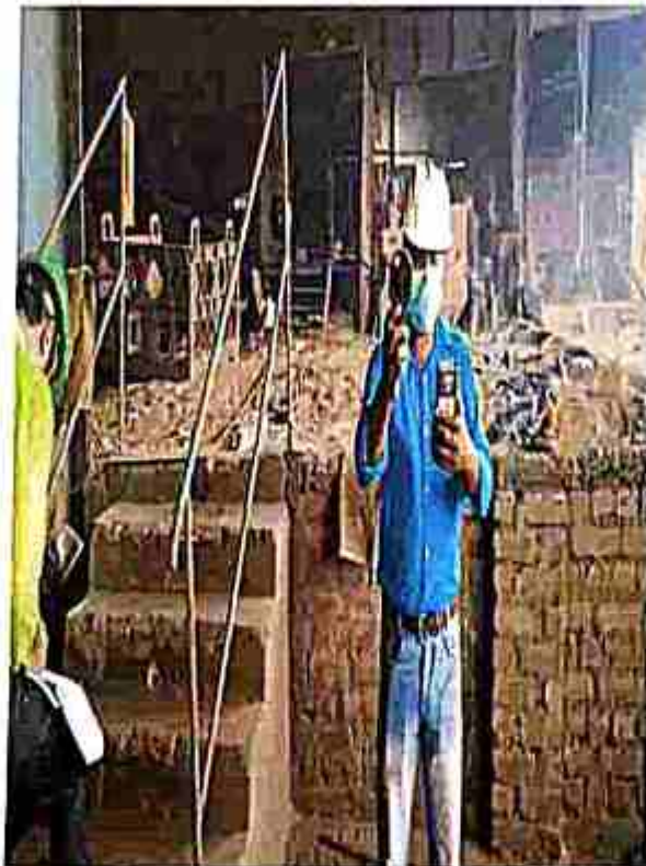
FERRO TAPING AREA
