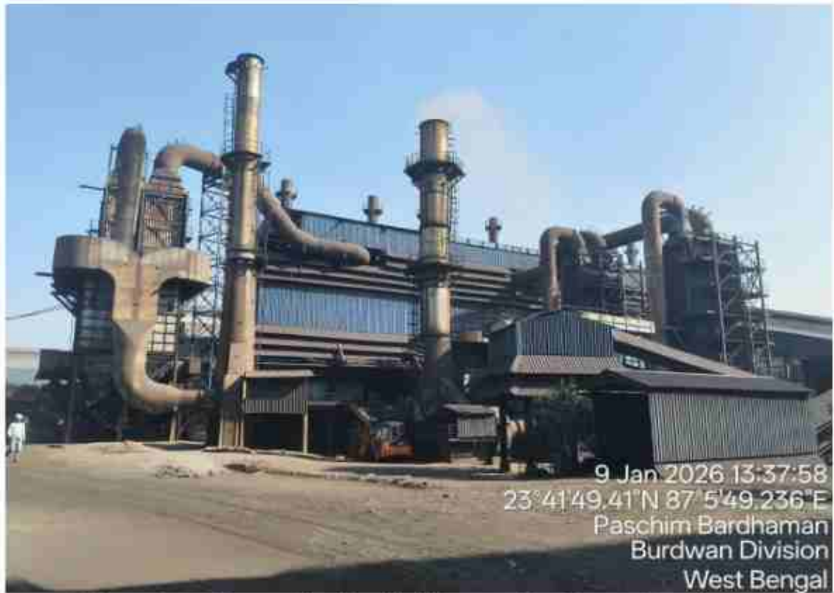
Pollution Control System (Bag Filter) for Submerged Arc Furnace (Ferro Division)
