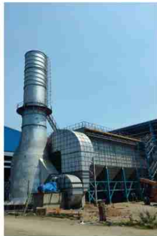
Bag Filter for Steel Melting Shop
