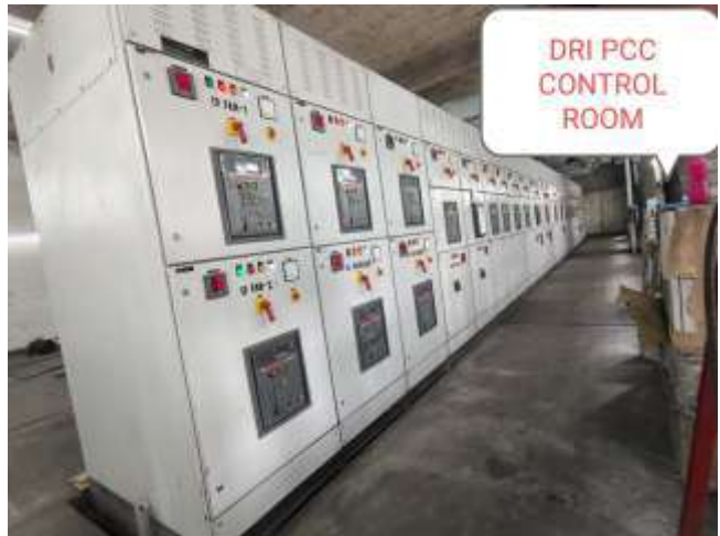
DRI 33KV HT SWITCHBOARD
