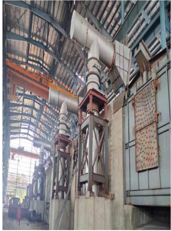
Induction furnace connected with primary hood
