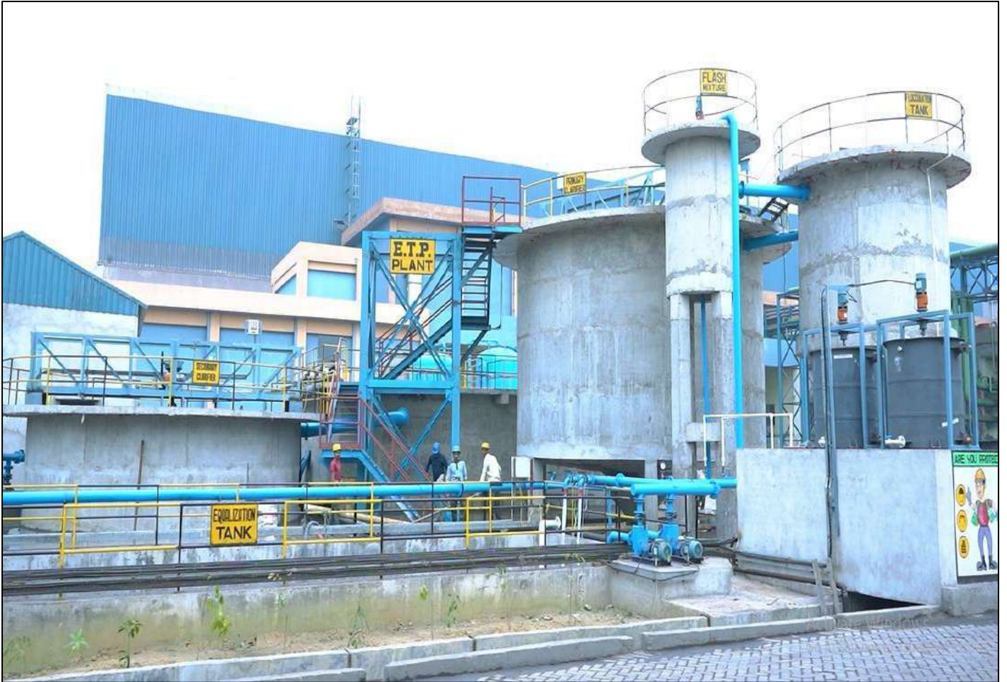
Effluent Treatment Plant (1540 KLD)
