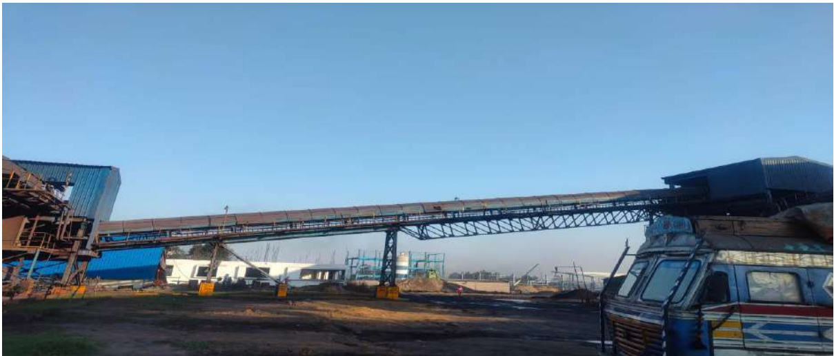
Closed Conveyor for raw materials handling
