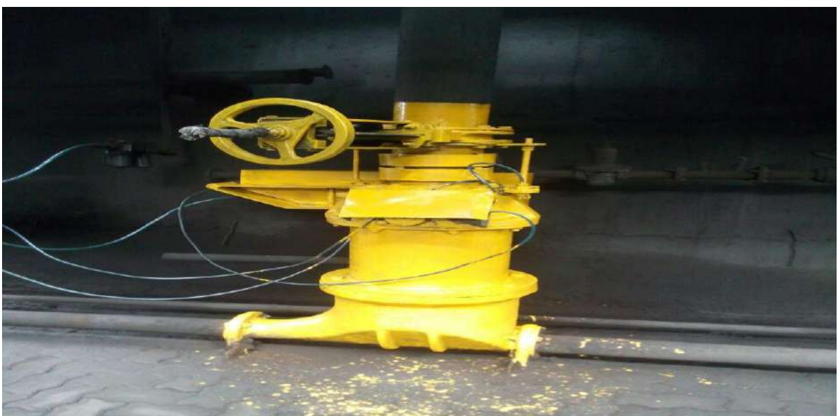
Pneumatic dust conveying system for fine dust
