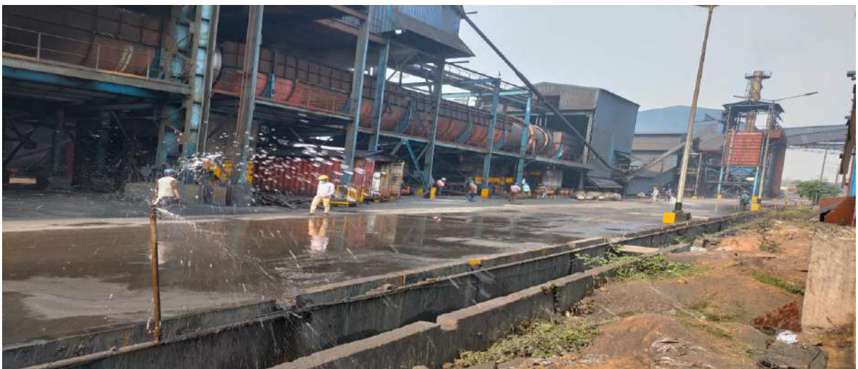
Water Sprinkler on road of plant site
