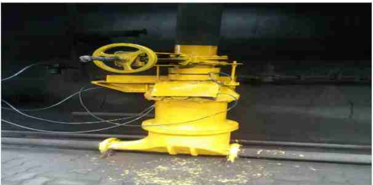
Pneumatic dust conveying system for fine dust
