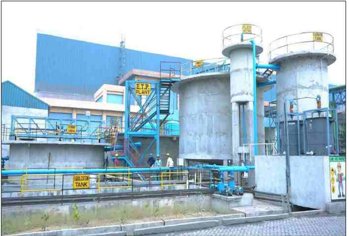
Effluent Treatment Plant (1540 KLD)
