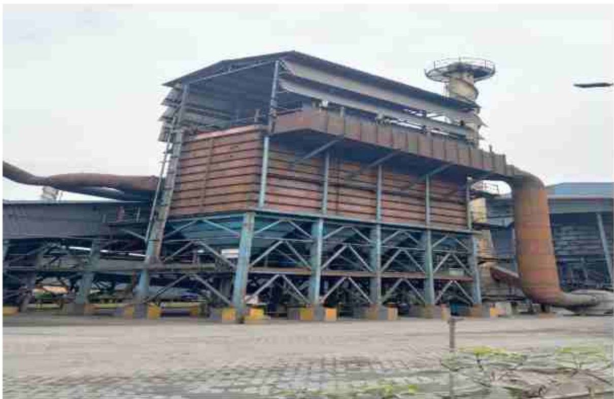
Bag filter connected with CD & I-Bin of 300 TPD DRI
