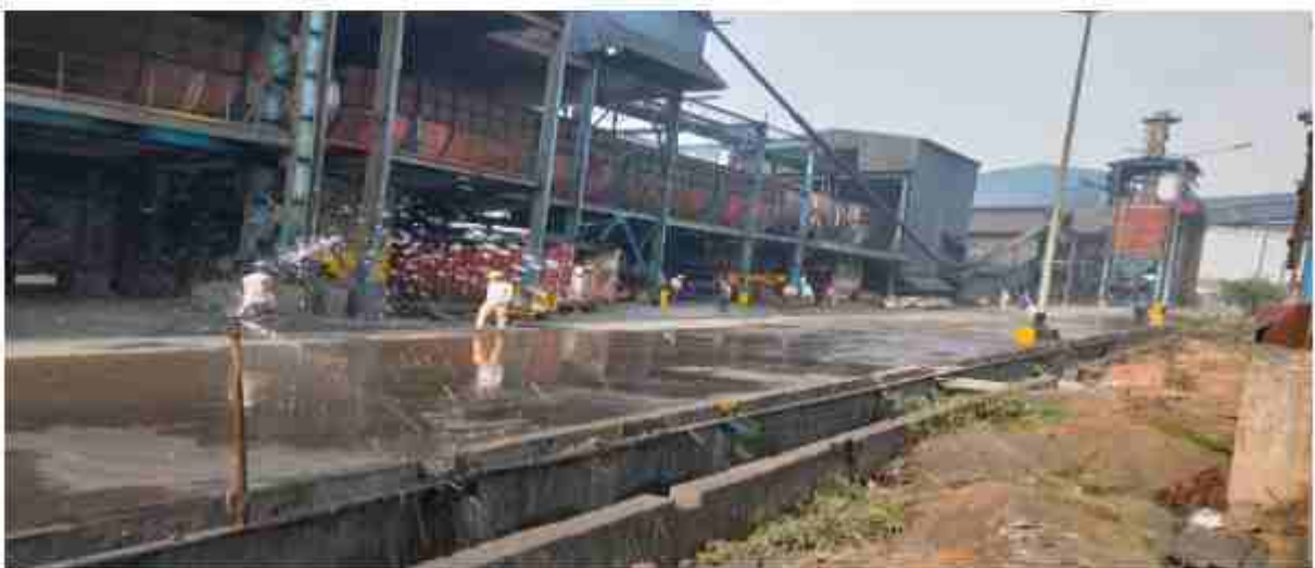
Water Sprinkler on road of plant site
