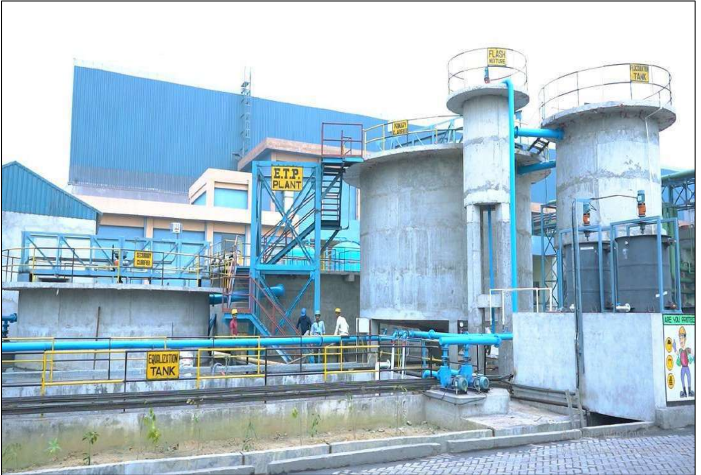
Effluent Treatment Plant (1540 KLD)
