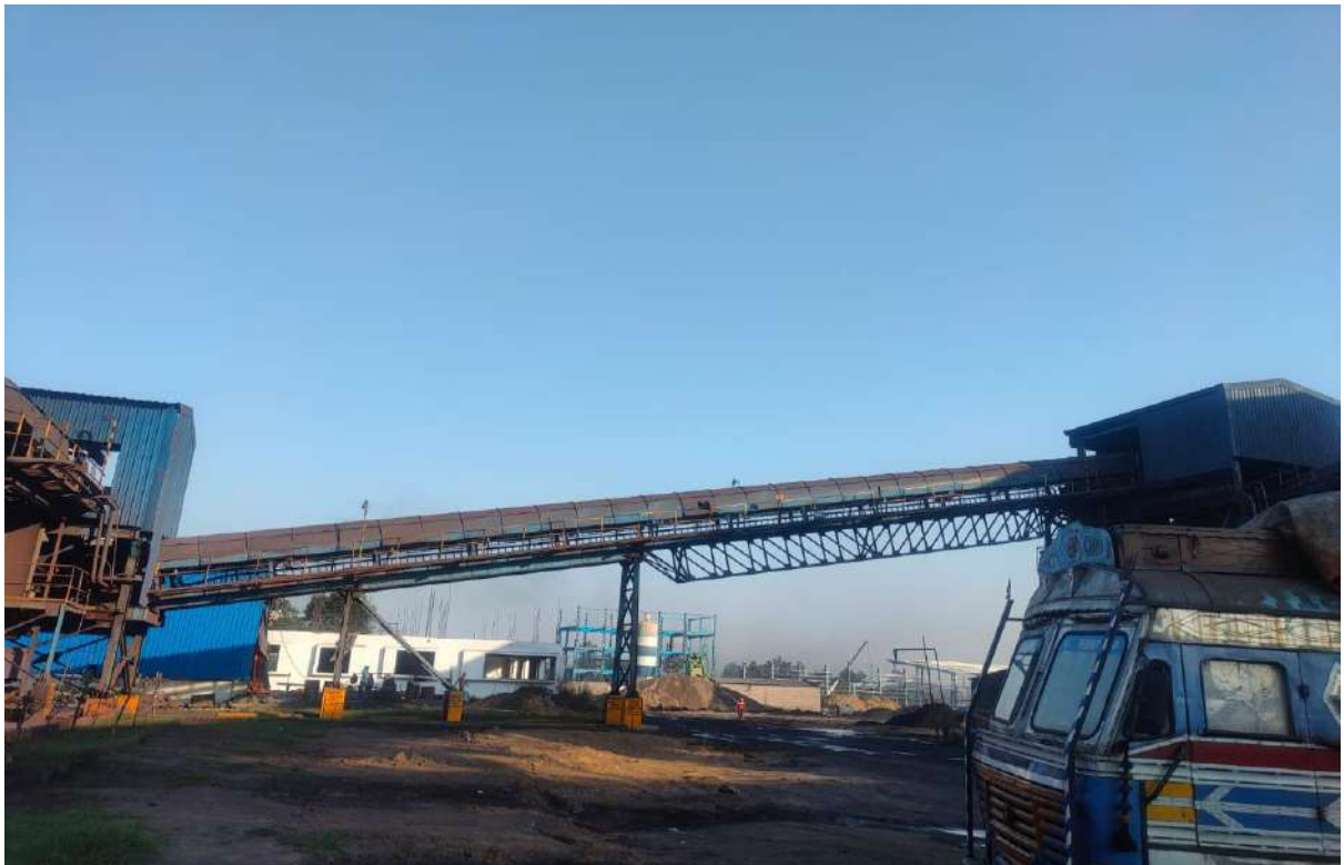
Covered raw material handling
