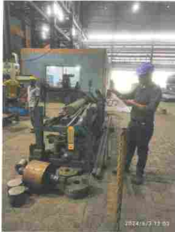
ROLLING MILL BILLET CHAIN TRANSFER AREA
