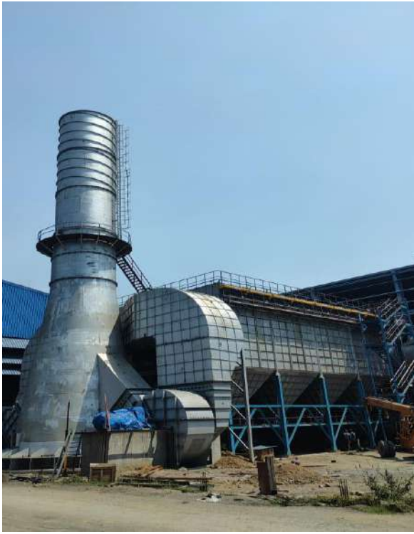
Bag filter with chimney connected with 6x20T Induction Furnace
