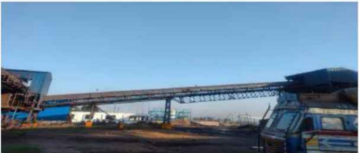
Closed Conveyor for raw materials handling
