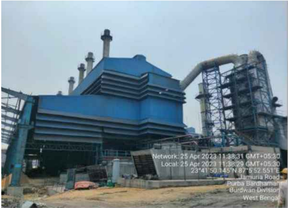
Bag Filter connected with 2x9 MVA SEAF
