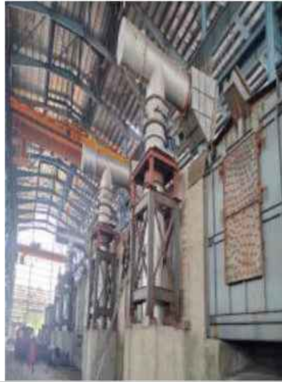
Induction furnace connected with primary hood
