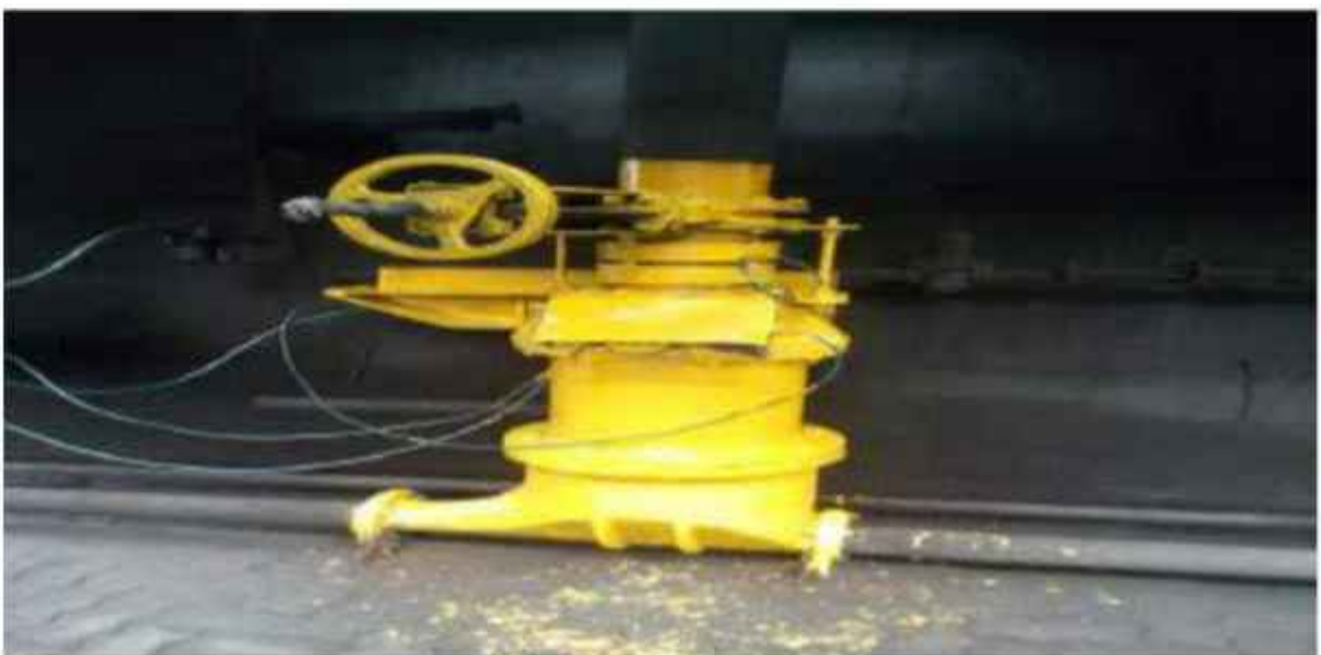
Pneumatic dust conveying system for fine dust
