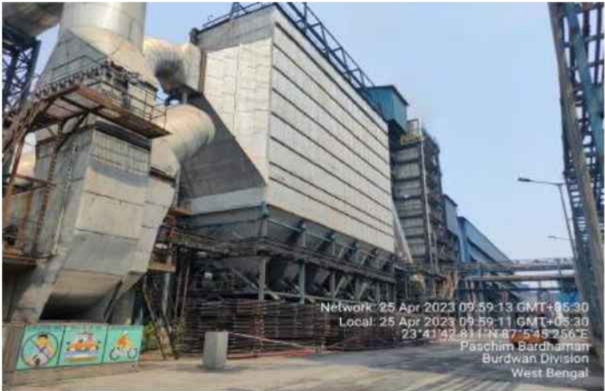
5 field ESP connected with 350 TPD DRI through WHRB
