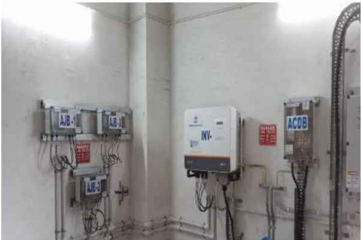
Photographs of Solar Power
