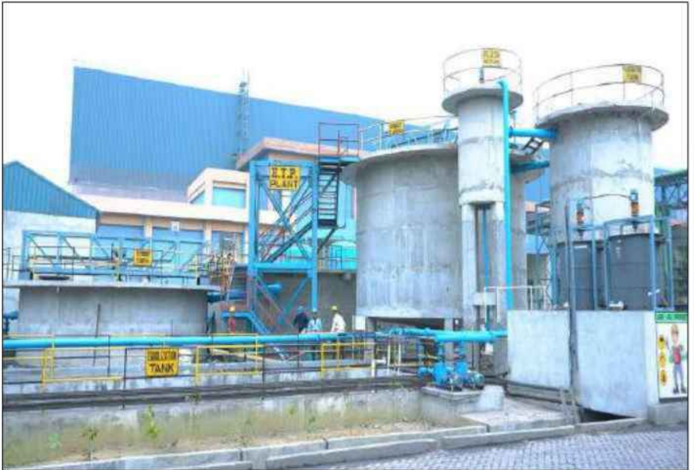
Effluent Treatment Plant (1540 KLD)
