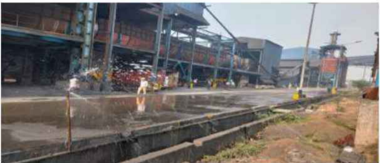
Water Sprinkler on road of plant site
