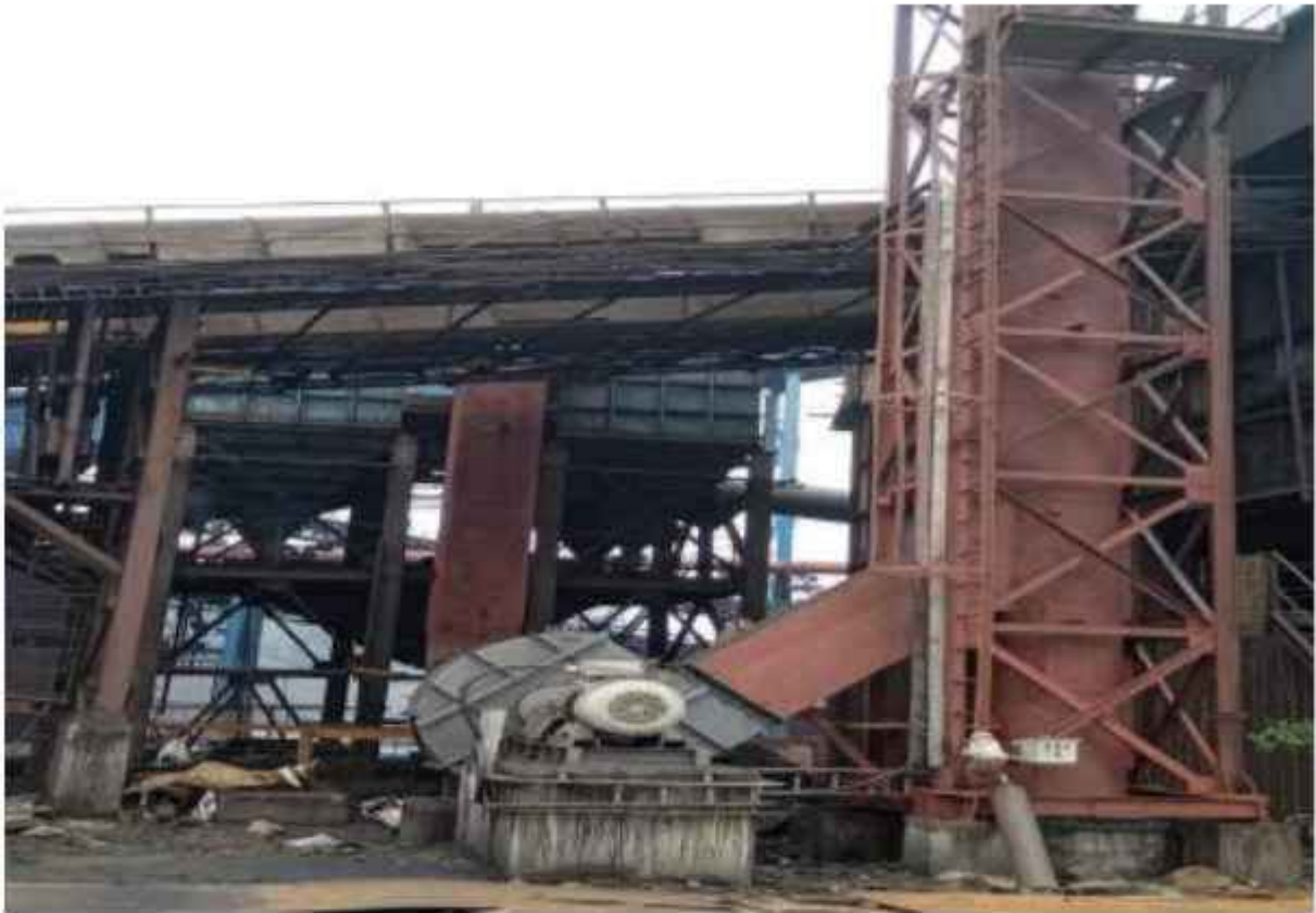
Bag filter connected with CD & I-bin of 600 TPD DRI
