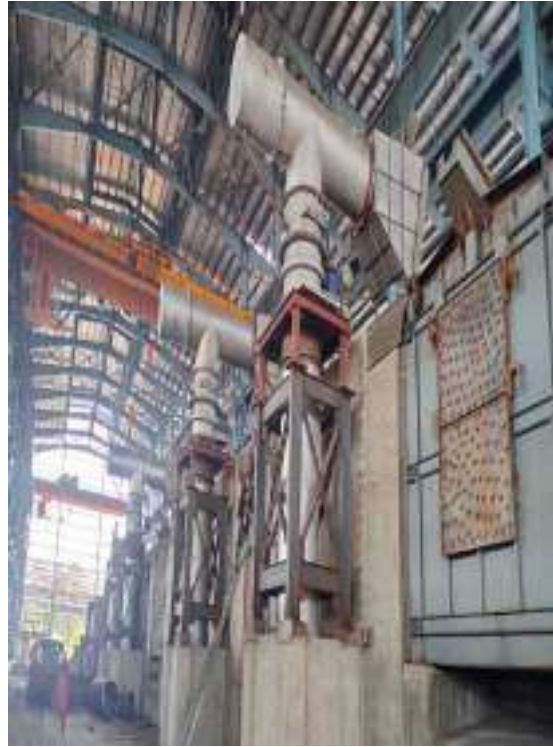
Induction furnace connected with primary hood
