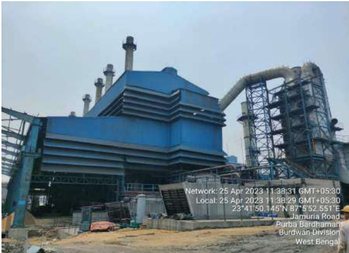
Bag Filter connected with 2x9 MVA SEAF
