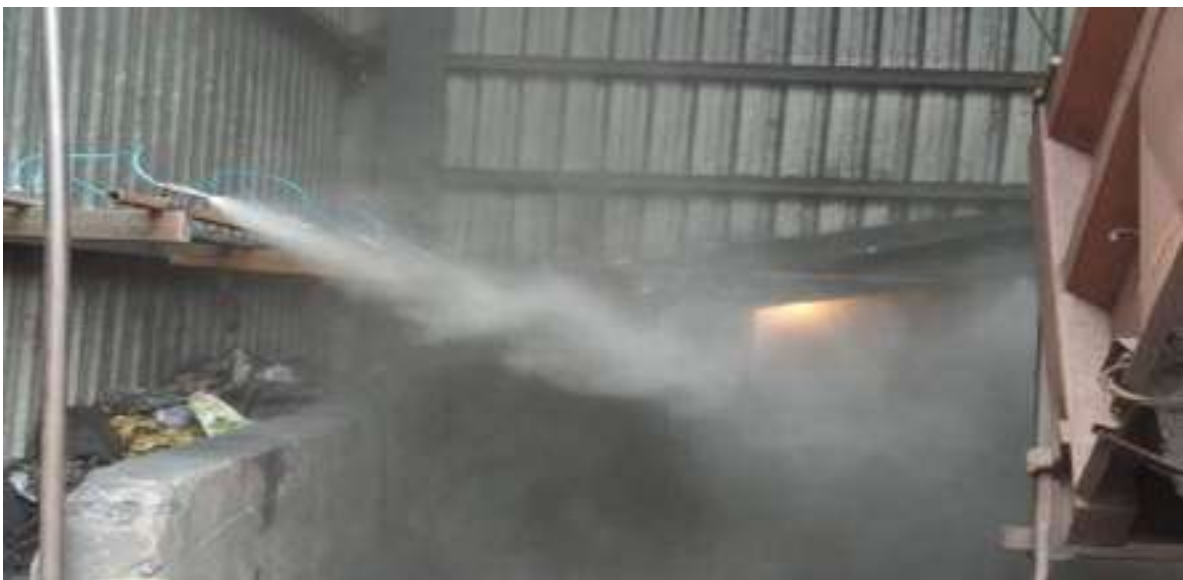
Dry fog system installed in coal handling system
