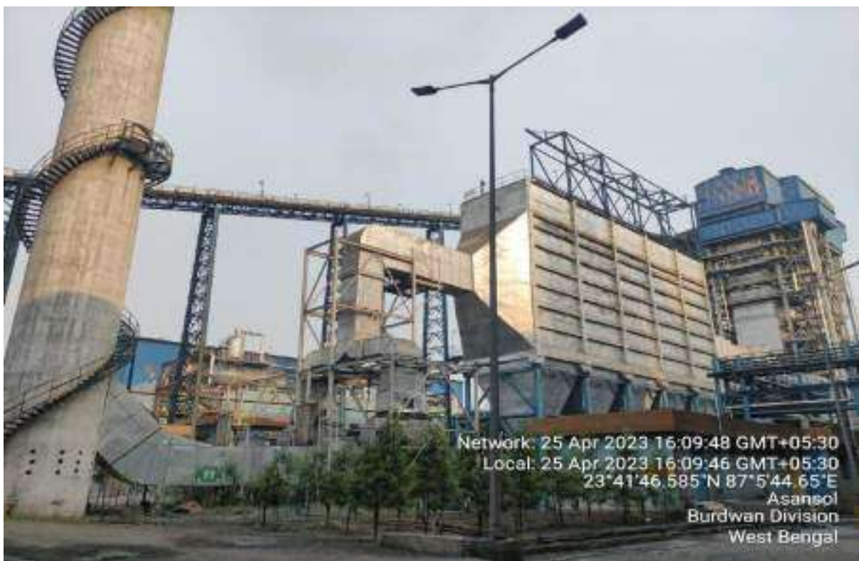
5 field ESP for CFBC Boiler
