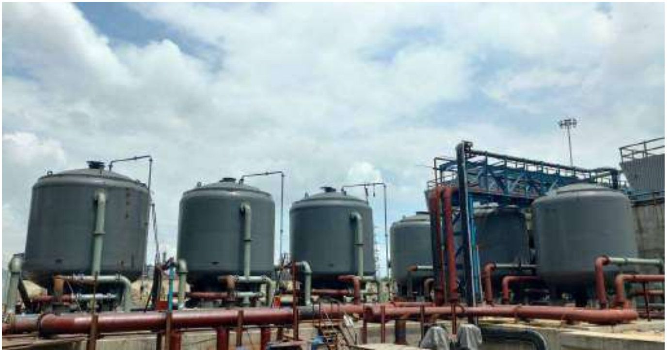
Filters for removal of Total Suspended Solids
