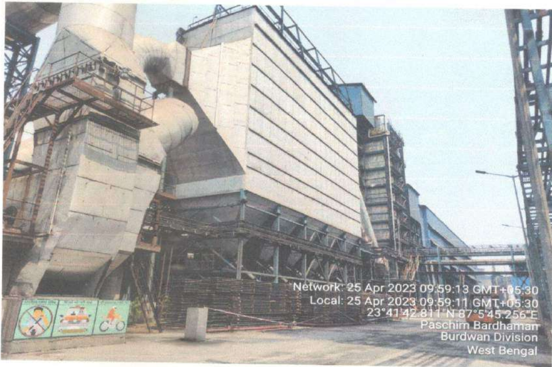
5 field ESP connected with 350 TPD DRI through WHRB
