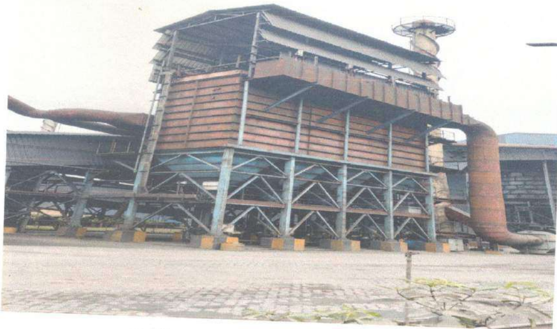
Bag filter connected with CD & I-Bin of 300 TPD DRI
