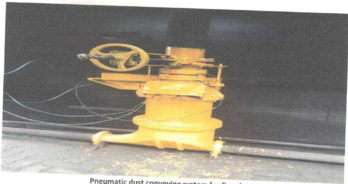
Closed Conveyor for raw materials handling
