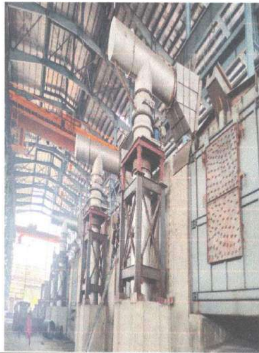
Induction furnace connected with primary hood
