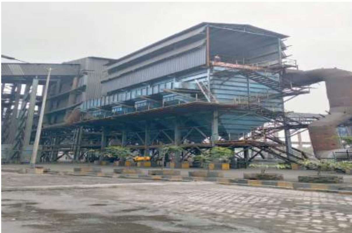
Bag Filter Connected with DRI 300 & 600 TPD (product separation & dispatch)
