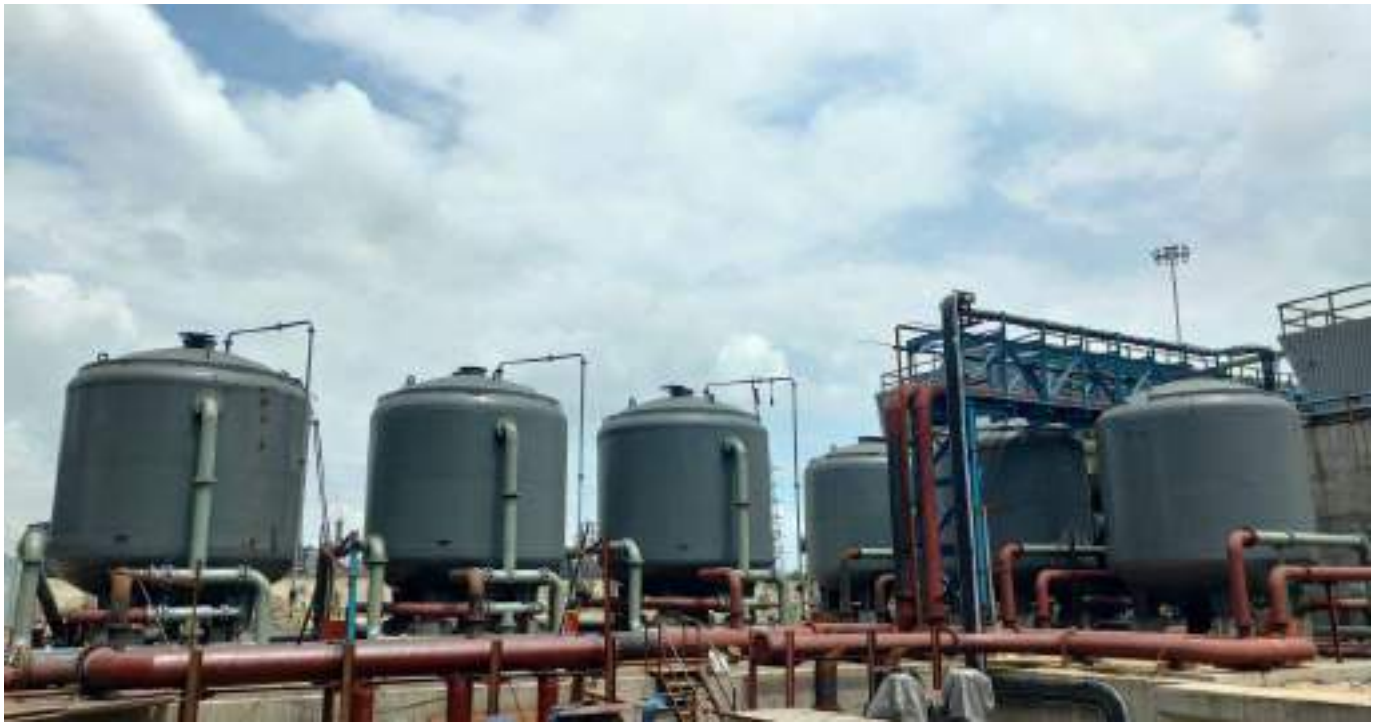
Filters for removal of Total Suspended Solids
