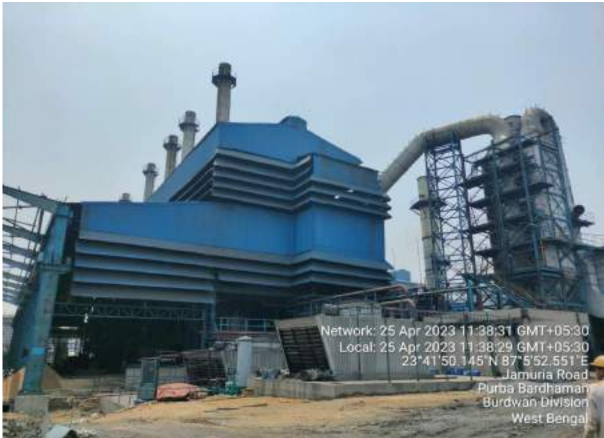
Bag Filter connected with 2x9 MVA SEAF
