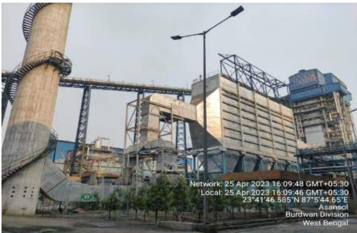
5 field ESP for CFBC Boiler
