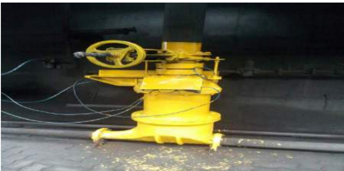
Pneumatic dust conveying system for fine dust
