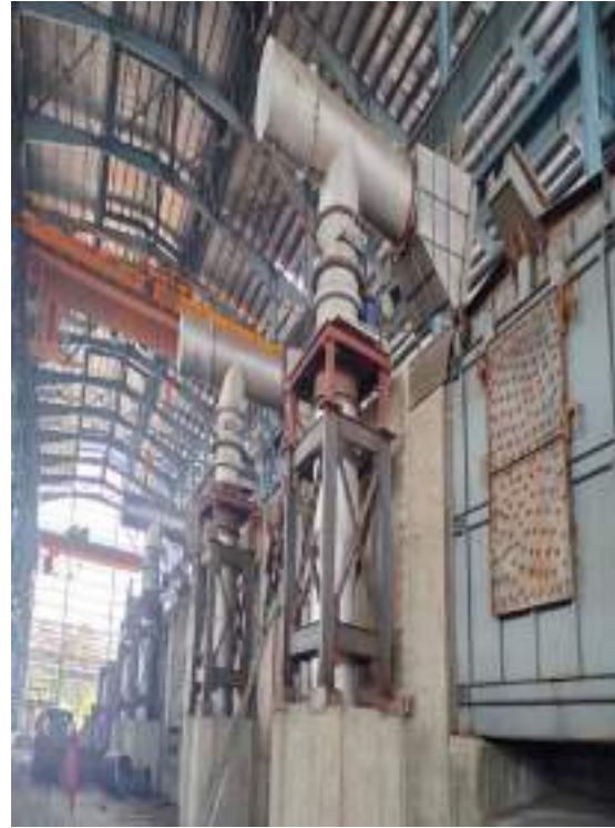
Induction furnace connected with primary hood
